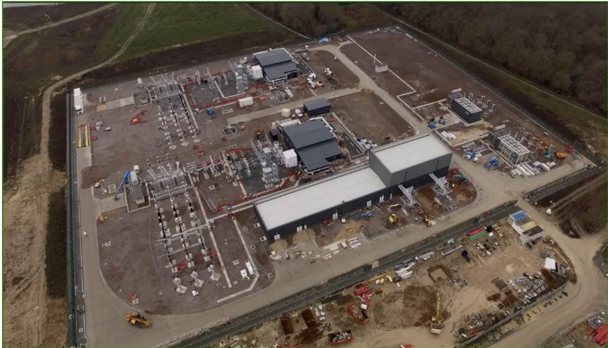
Plate 6.1 Example Layout of the Onshore Substation (example taken from construction of East Anglia ONE substation)
