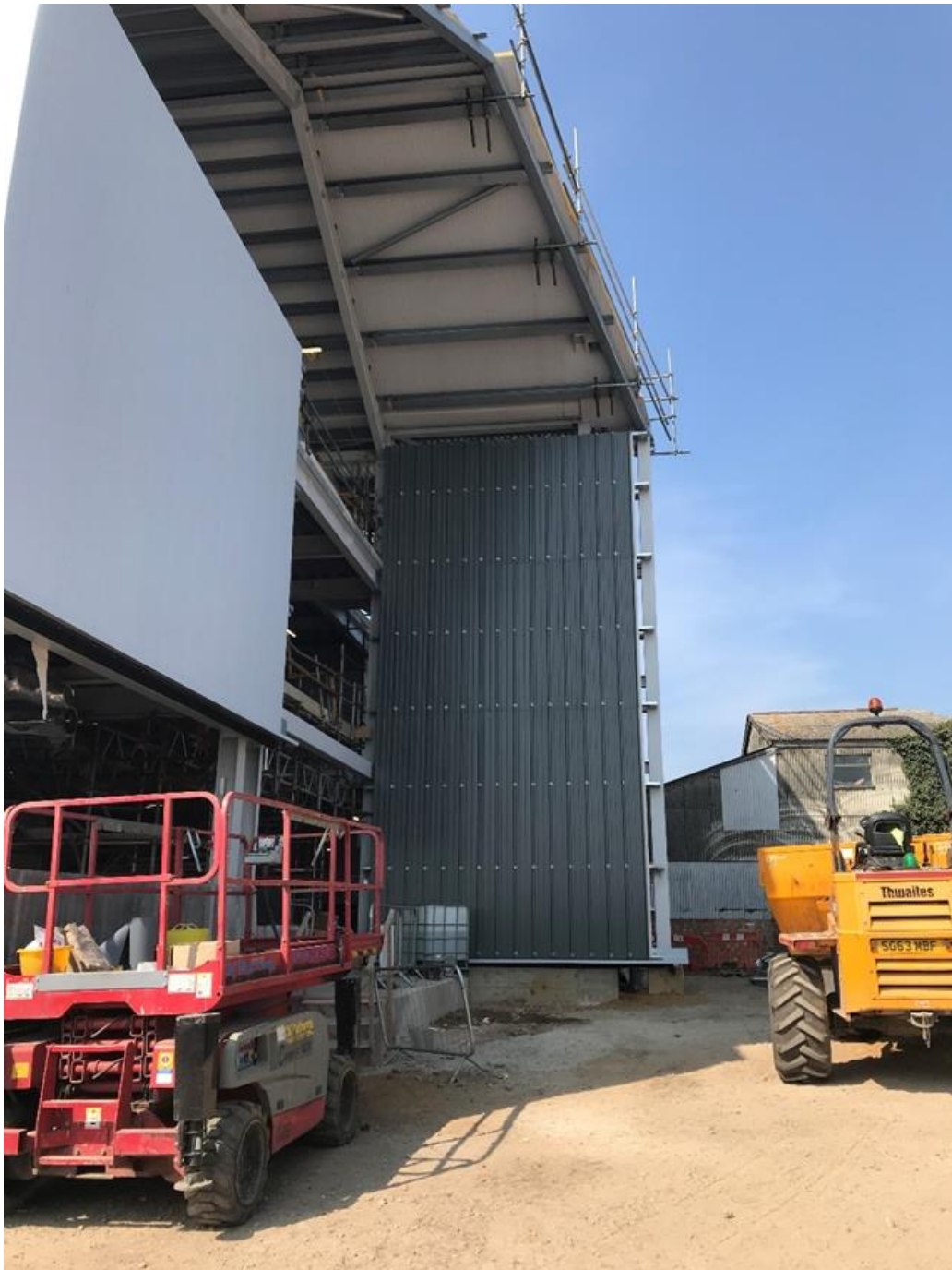
Plate 6.2 Example of dark grey composite cladding used on a substation office building (example taken from construction of East Anglia ONE substation)
